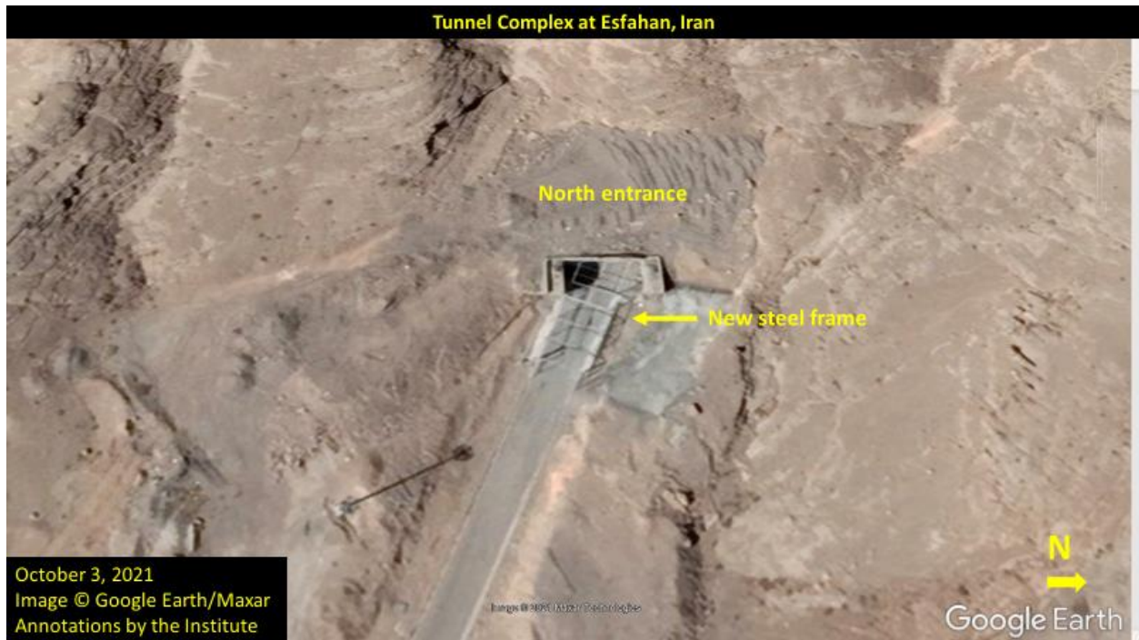
Figure 4. The North entrance tunnel in October 2021, after a steel frame was added to the entrance area.
