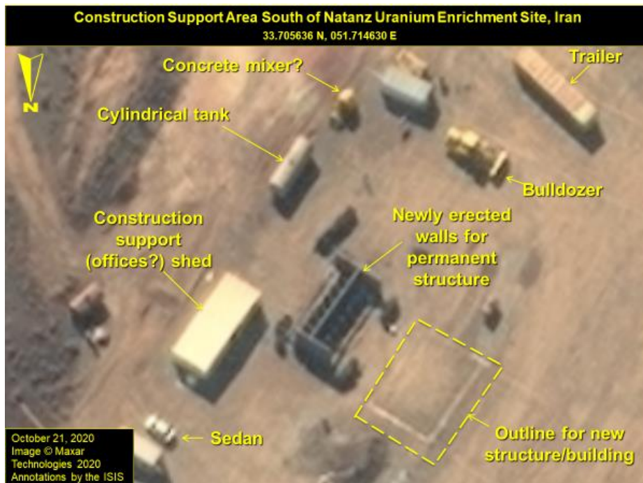
Figure 1. A close-up of the construction staging area and possible future support area for the underground centrifuge assembly.
