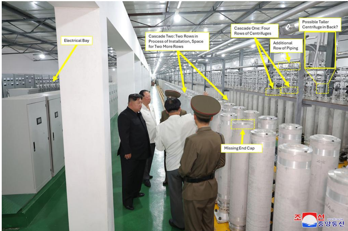
Figure 12. A second, very long enrichment hall visited by Kim Jong Un. Electro-pneumatic valves on the dump line can be seen that look new. Pressure gauges are not visible, but they may be on the opposite side of the four-row cascade.
