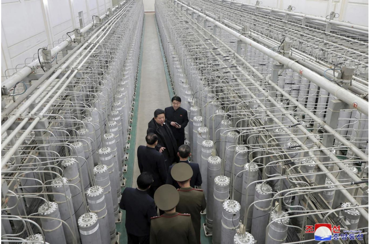
Figure 17. A partial view of a narrow cascade hall, likely the original Yongbyon hall. This image shows the full width of the room, i.e. both walls, if not its full length. A door is visible on the left. Two rectangular block-shaped pressure gauges, with Pirani gauges or pressure transducers, can be seen in the middle-right lower part of the image.
