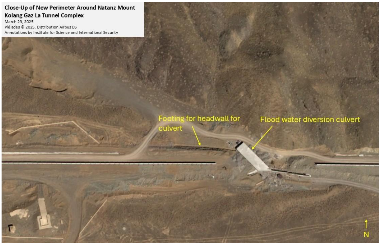
Figure 6. A close up of the construction of a water diversion culvert on the south side of the perimeter.
