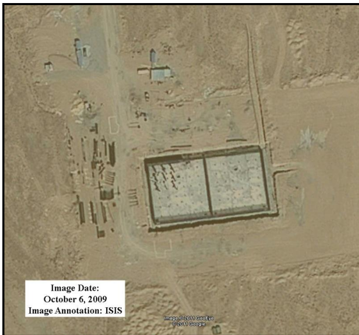
Figure 8. October 6, 2009 satellite image shows building under construction at southern end of Ardakan site.
