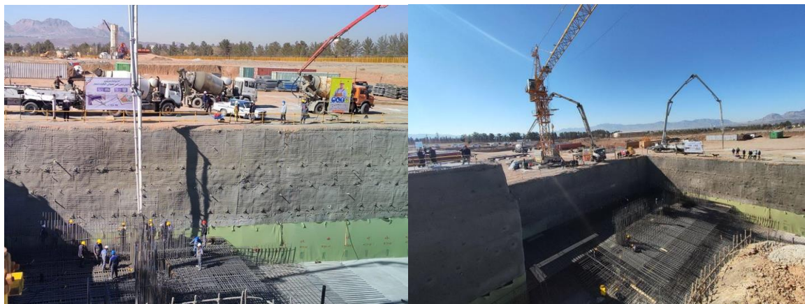
Figure 2. Ground image of the construction of the Esfahan research reactor in early February, 2024. 3
