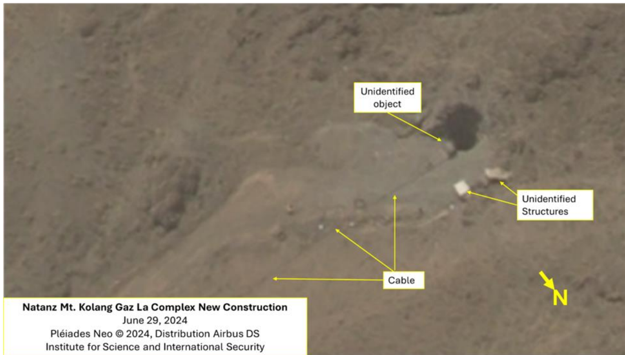
Figure 4. The construction site of the probable ventilation shaft on June 29, 2024. An additional unidentified object appeared.
