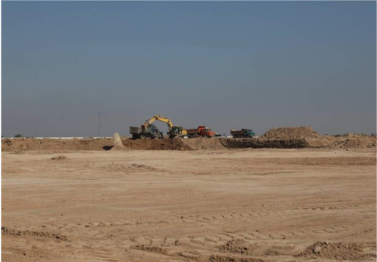
Figure 3. Ground image of the Darkhovin site in 2023, showing site clearing that matches activity in Figure 1. Source: Tasnim News, “The end of the excavation of the nuclear island of the 300 MW Karun nuclear power plant / the start of concreting of the power plant in the fall of 1403.”
