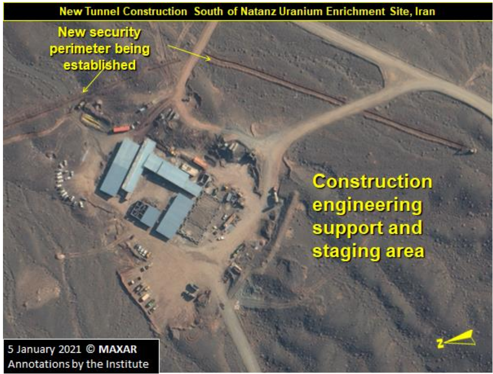
Figure 2. In addition to construction equipment, the construction staging area features several buildings and a partly-established security perimeter.
