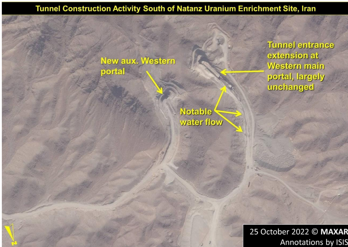
Figure 7. Water flow at the western main tunnel portal.
