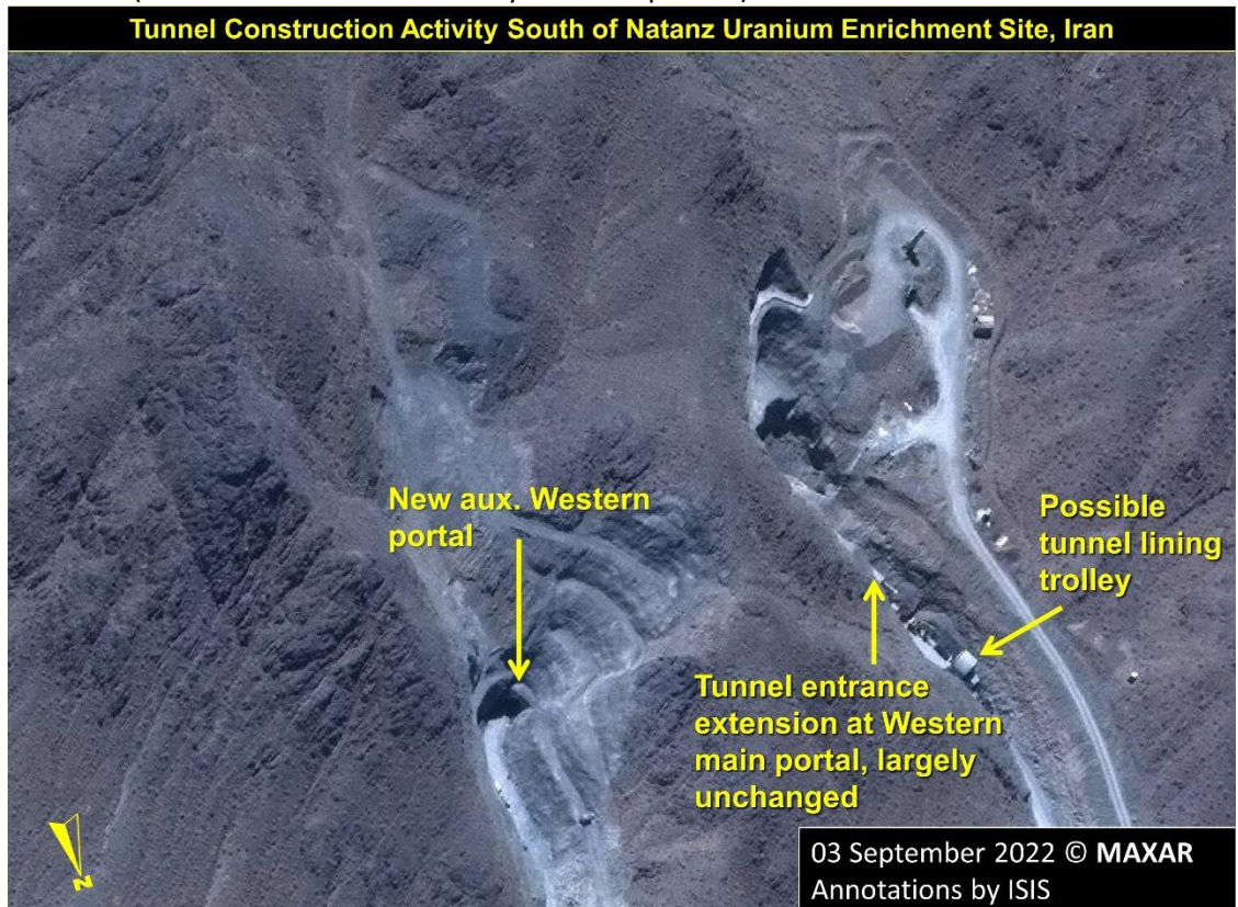
Figure 3. A close-up of the new tunnel entrance shows the entrance completed as of September 2022.
