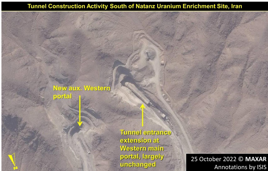
Figure 5. The pre-existing western tunnel entrance also features a new entrance extension, likely to be covered by earth in the future. It appears largely unchanged since May 2022.
