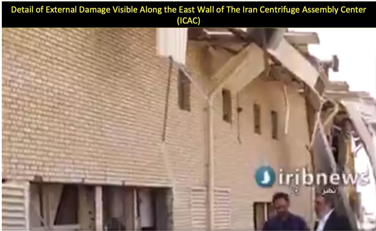
Figure 3. Closeup of the east wall of the ICAC showing severe roof damage.
