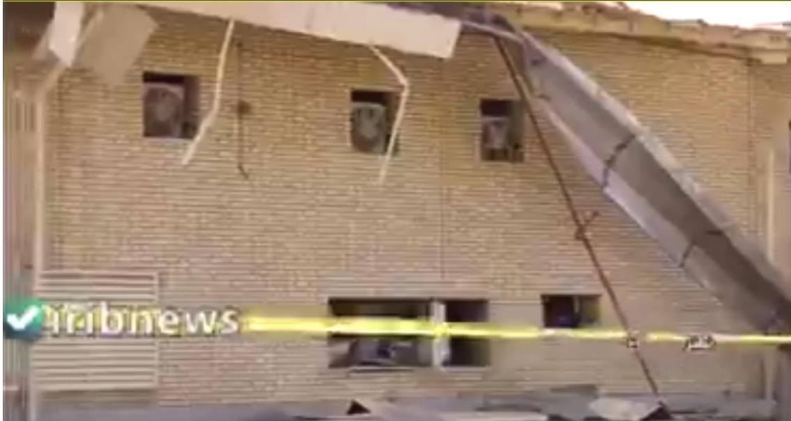
Figure 4. Closeup of the east wall of the ICAC showing the building had been cordoned off with yellow tape.
