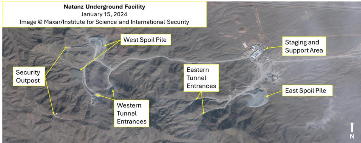
Figure 1. A January 2024 overview of the tunnel complex under construction just south of the Natanz Fuel Enrichment Plant.
