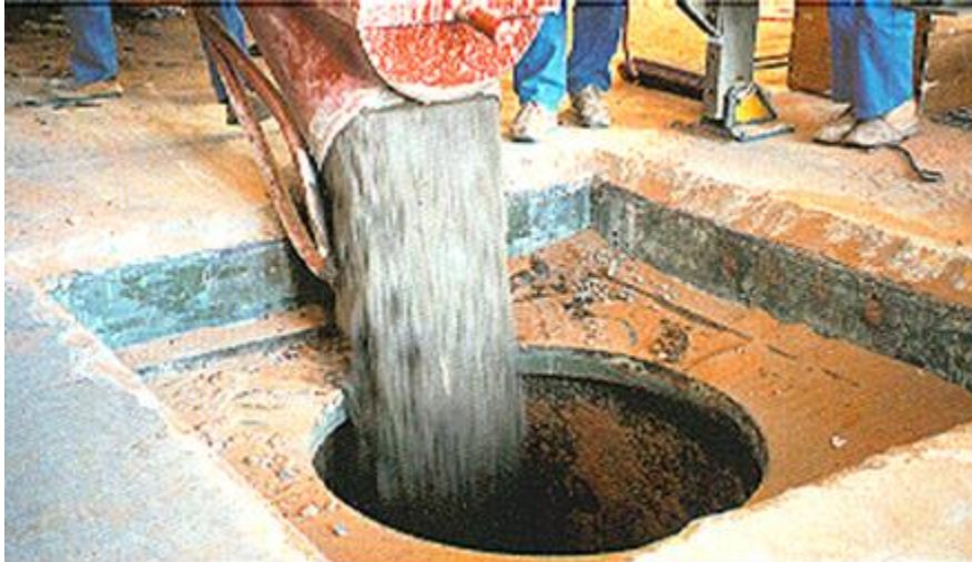
Figure 5 Casting concrete in test shaft 1 inside the shade (July 1993). Source: IAEA, Against the Spread of Nuclear Weapons: IAEA Safeguards in the 1990s , http://www.iaea.org/Publications/Booklets/Safeguards/pia38e14.html
